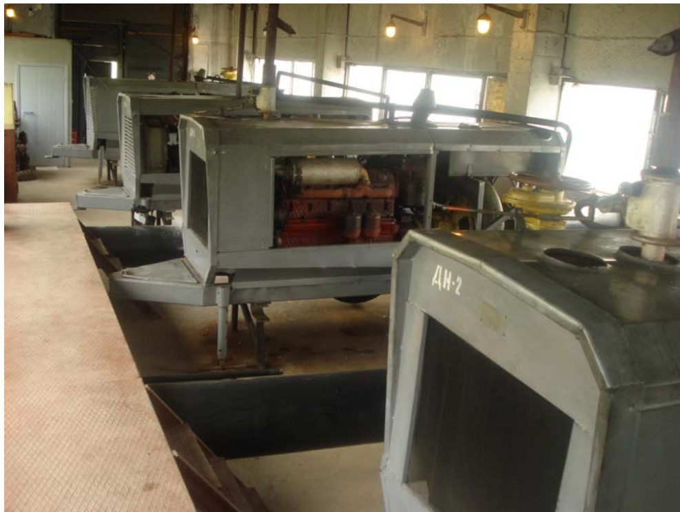
Picture 4. Diesel Pumps of Essential Service Water System
