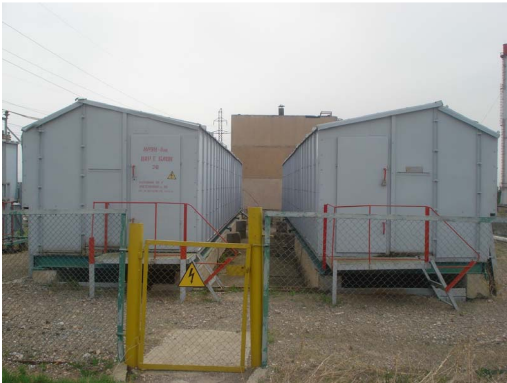
Picture 3. Auxiliary Cooling System
